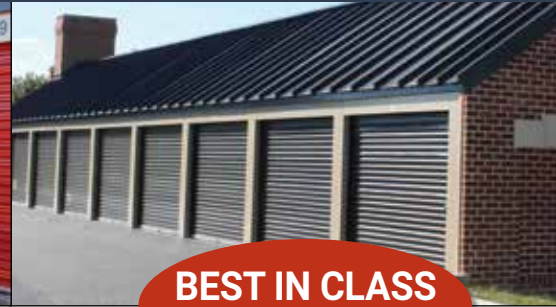
ALL DOORS ARE WIND RATED
